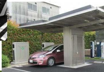
Right bottom: A battery system utilizing waste batteries of PHVs at Ecoful Town
