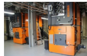
↑Wood biomass boilers
