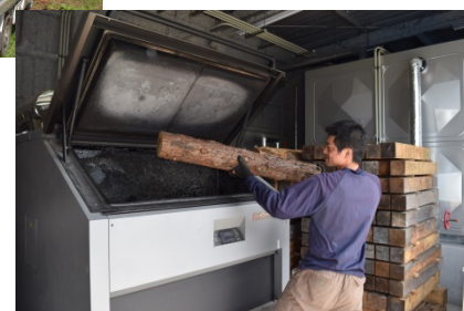
↓Woody (firewood) biomass boiler
