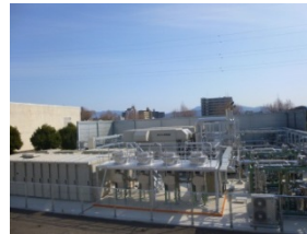
Matsuyama City Central Purification Center Digestion gas power generator
