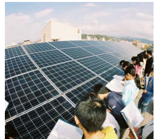
Viewing a photovoltaic system installed on the rooftop of an elementary school
