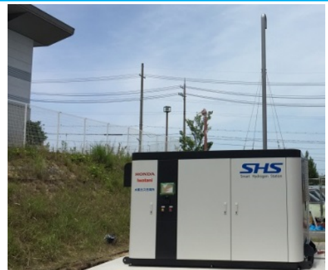
Kobe Renewable Energy Hydrogen Station
